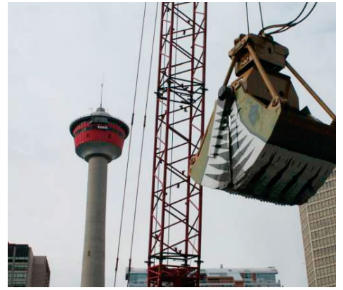
The clamshell bucket being used to excavate the future site of the Telus Sky building hangs from its crane with the Calgary Tower in the background.
